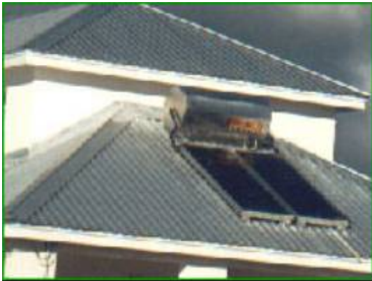
Solar water heating system installed in Barbados
